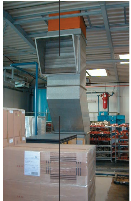
air outlet for excess compressor heat
